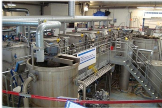
Figure 10. Line 1 of Hammarby Sjöstadsverk that was used in this test. Line 1 was operated as a conventional WWTP with chemical phosphorous removal.
