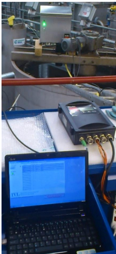
Figure 4. Cerlic CBX test setup in Line 1.
