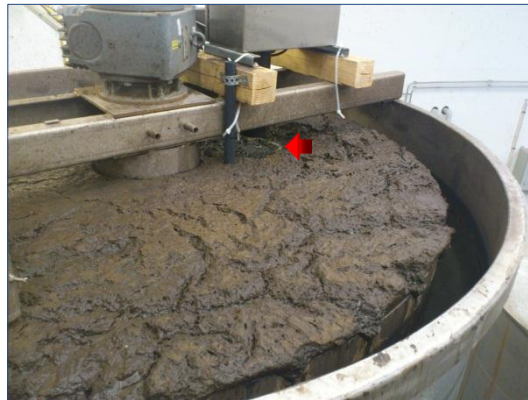
Figure 14. Sedimentation basin with thick top sludge layer and visible dilution near the sensor that is generated by the automatic cleaning of the CBX sensor.
